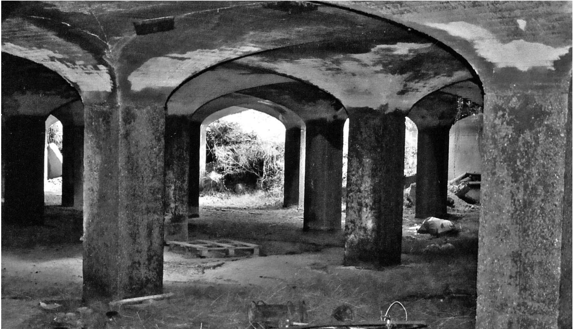
Partially collapsed underground filtration cell
